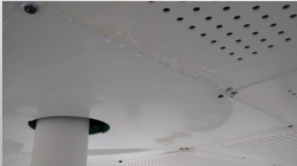
Water condensation from UDAF system
