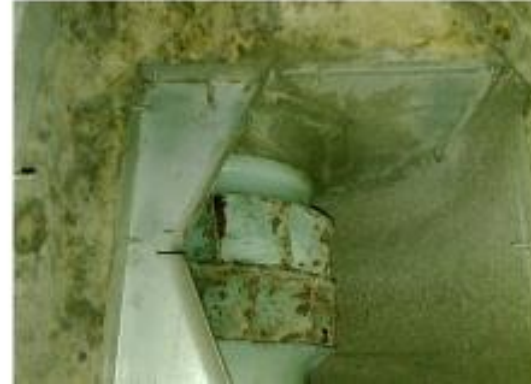
Air handling units
